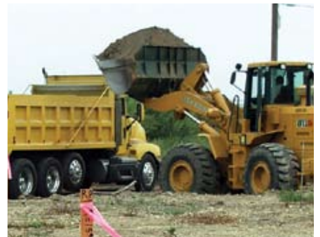
Funded by a grant from the Los Angeles County Metropolitan Transportation Authority, the new parking area will provide space for 44 vehicles and 2 school buses along with bicycle racks.
